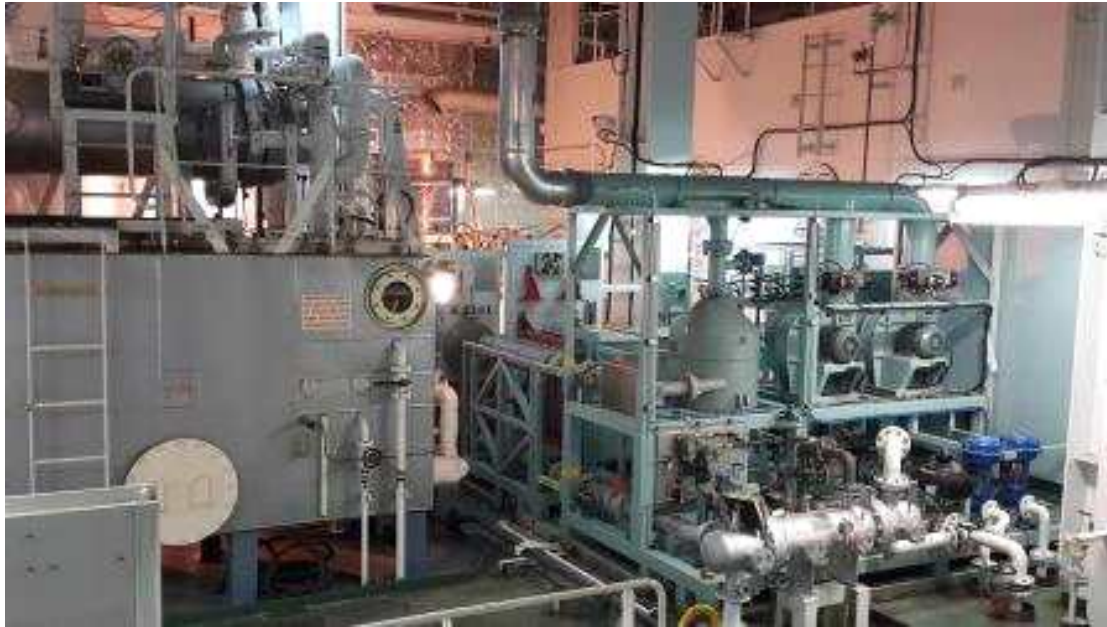
[Fig. 44] Example for typical field installation of BWMS hired technology of Electrolysis (Side-stream type)
