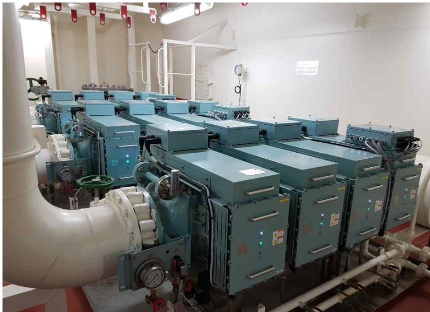
[Fig. 43] Example for typical field installation of BWMS hired technology of Electrolysis (Full-flow type)
