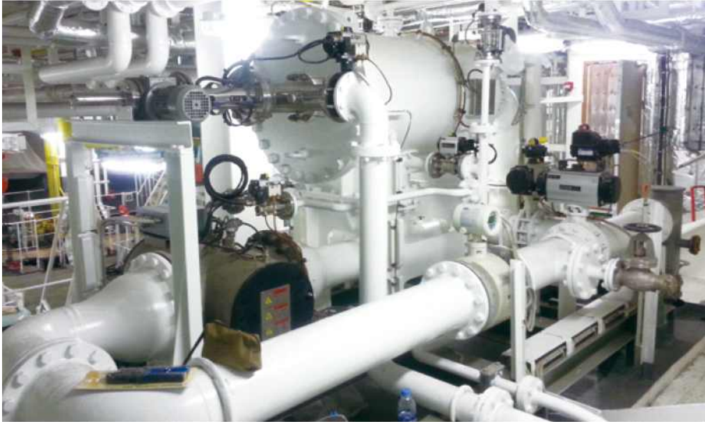
[Fig. 42] Example for typical field installation of BWMS hired technology of UV
