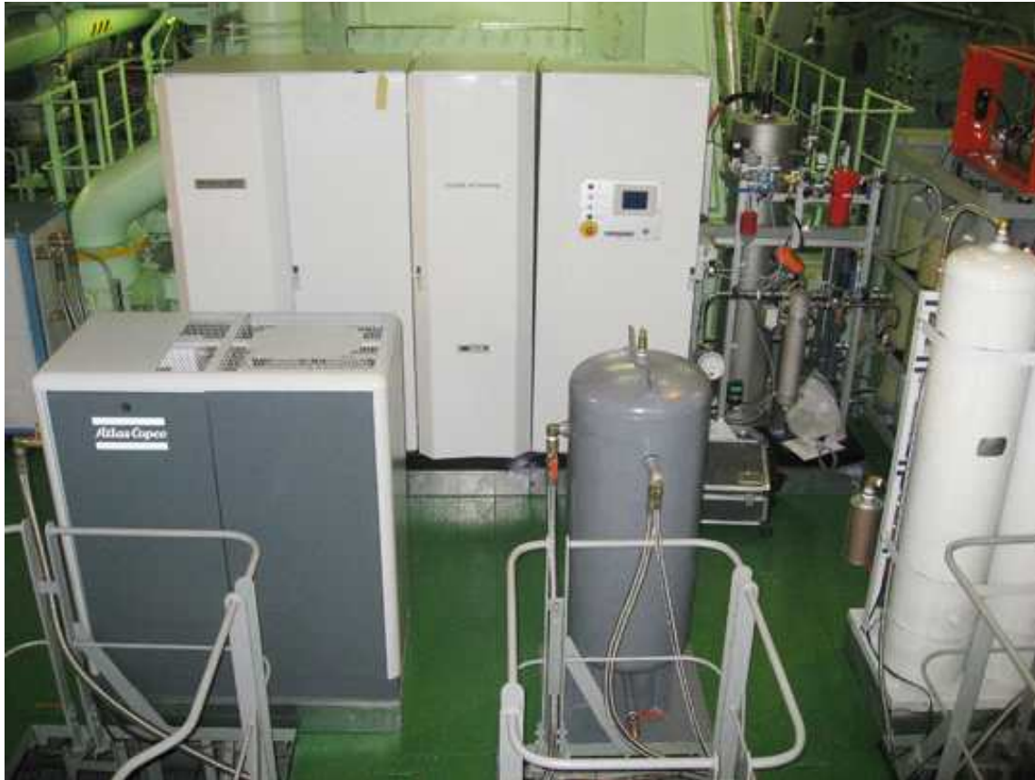
[Fig. 45] Example of typical field installation of Ozone system
