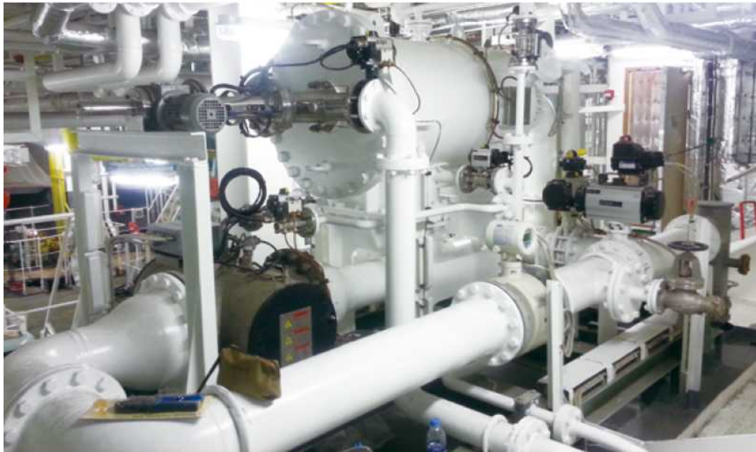
[Fig. 42] Example for typical field installation of BWMS using UV technology
