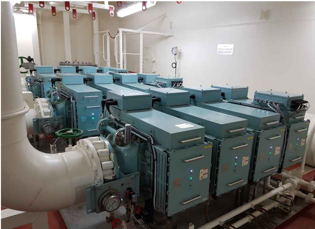
[Fig. 43] Example for typical field installation of BWMS using Electrolysis technology (Full-flow type)
