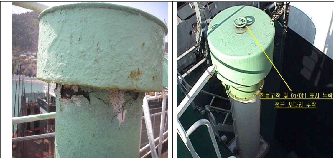
8. Examining the ventilators and air pipes, including their coamings and closing appliances (202. 1 (6))
