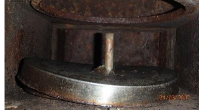
Warped Disk/Missing gasket
