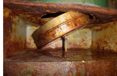
Post too short, disk slipped off
