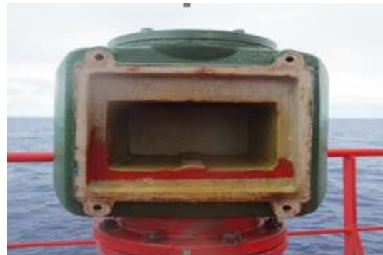
Missing disk and post
