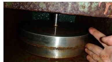
Broken Post/missing gasket
