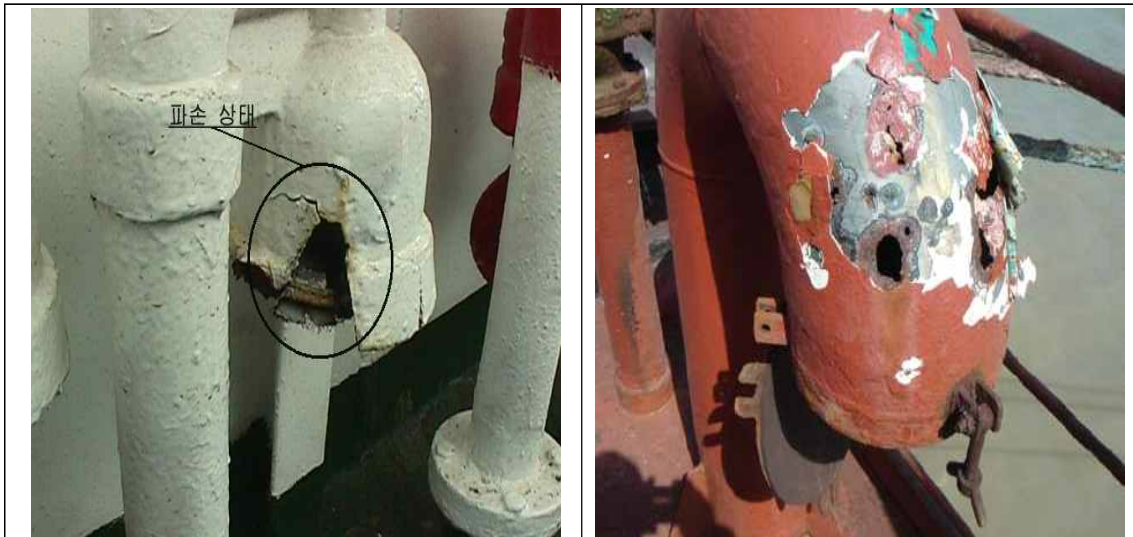
7. External examination of all air pipe heads installed on the exposed decks (202. 1 (1) (g))
